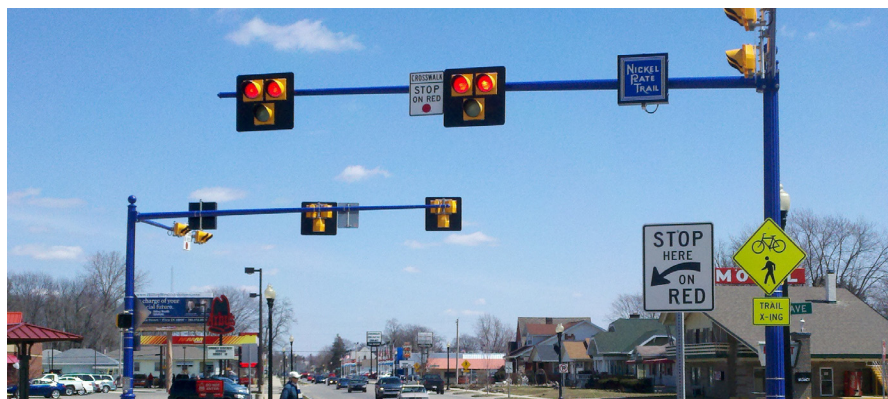
Signals and warning devices
