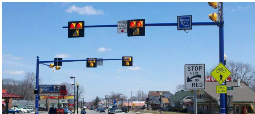
Signals and warning devices
