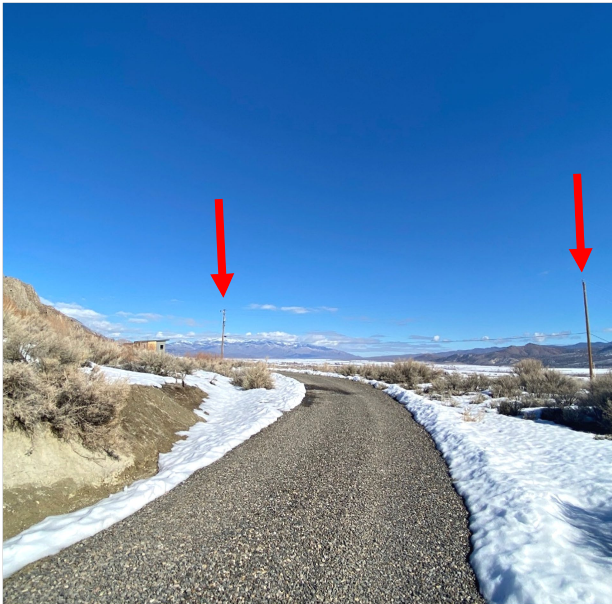
FIGURE 4: Olson Residence from the south looking north. Picture shows the two poles from the driveway. The line is undergrounded the last 180+ feet from the second pole to the residence.
