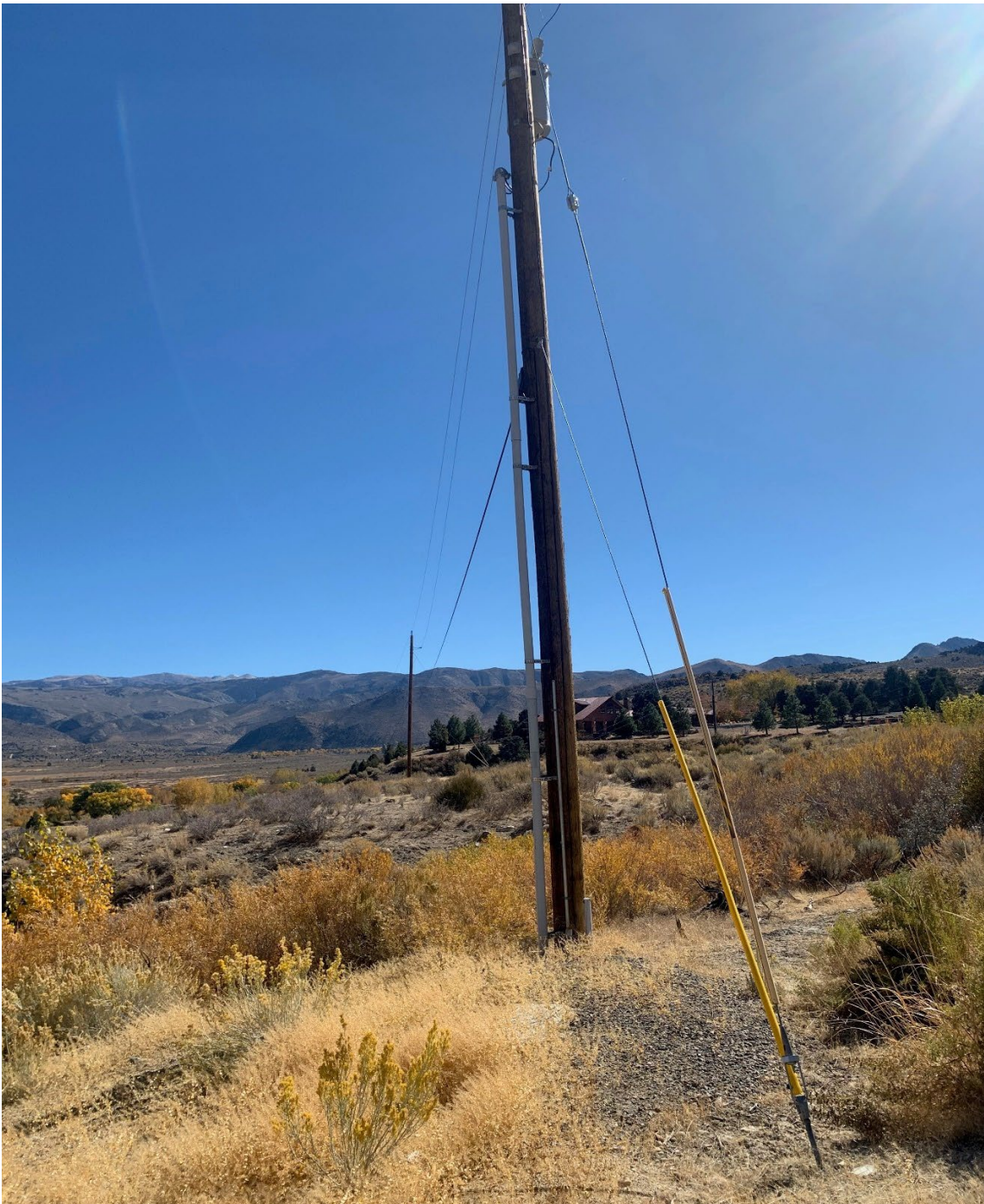
FIGURE 6: Picture of both power poles looking from the second service pole, closest to Olson Residence, looking across the steep riparian drainage toward the southeast.
