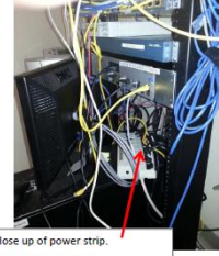
Close up of power strip.
