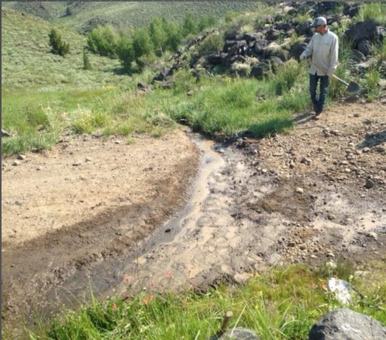
Spring erosion along the Burcham Flat Road
